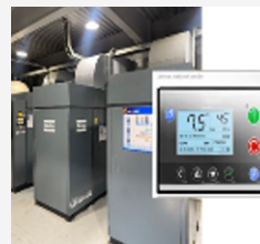
Compressor Air Pressure Adjustment
